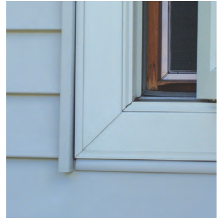
Finished windows such as these are common and are an invitation for water and insects.
